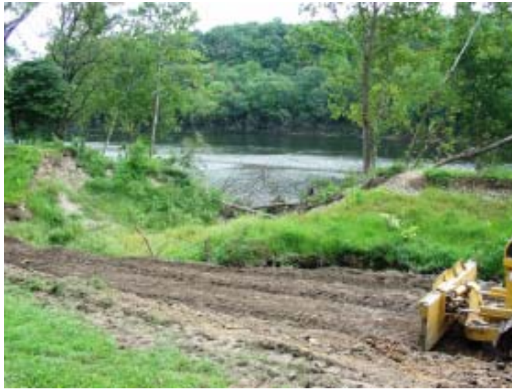
The towpath bank break south of Easton is creeping into the neighbor's lawn.
